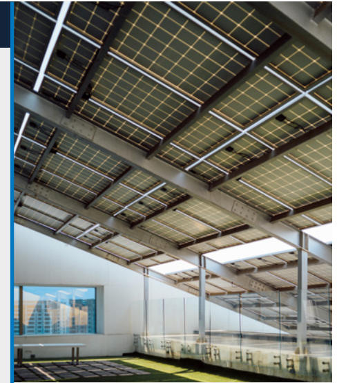
Solar panels on roof of De Beers Group Industry Services Building, Surat.
